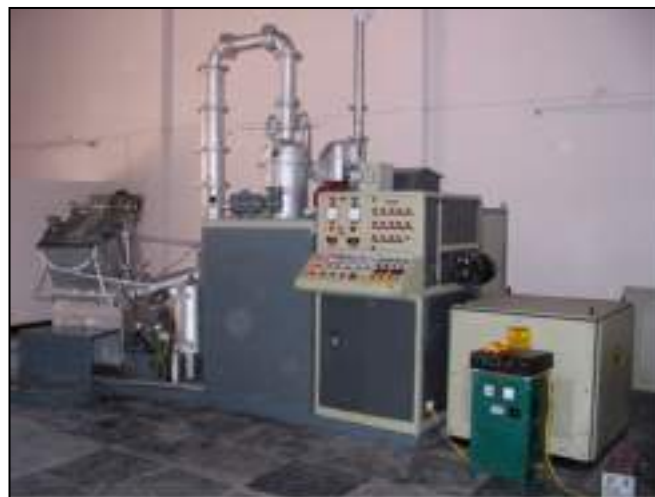
Figure 2: 15kg/hr. Plasma Pyrolysis System installed at Goa Medical College, Bambolim, Goa
