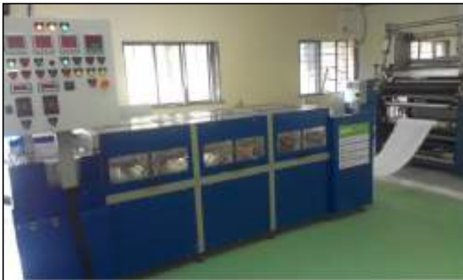
Figure 3: Atmospheric Pressure Air Plasma system installed at MANTRA
