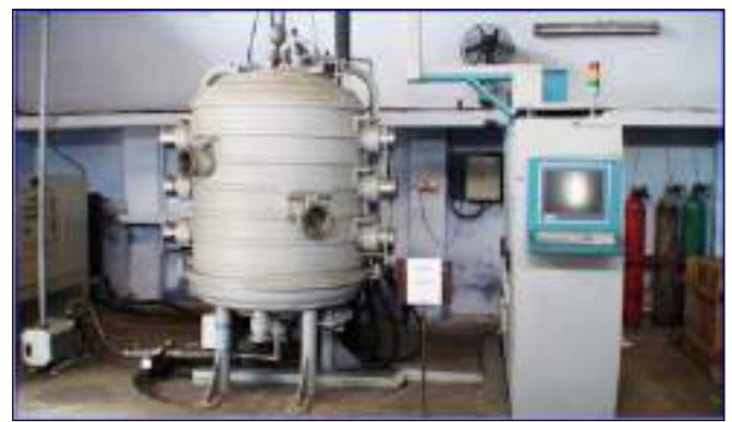
Figure 4: Plasma Nitriding system installed at CTR, Ludhiana by our licensee partner.
